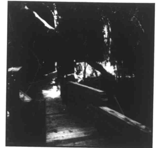
Stacks of lumber waiting to be put in place line the boardwalk at Hoo-Hoo Park. The boardwalk is the highlight of the project and is nearly one fourth done. When finished, the boardwalk will connect the nature center, the Indian River, and the parking lot, with crossover walks at intervals along the way. There will be a total of 3500 feet of boardwalk.
